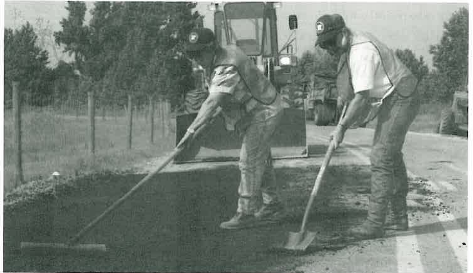
District 5 Searcy Maintenance Crew Leader Irma Collins and Single Axle Truck Driver JoAnn McWilliams complete an asphalt repair.
